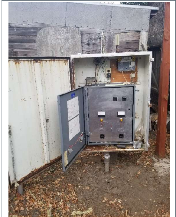
Photo 8. Lift Station 2 Cabinet
