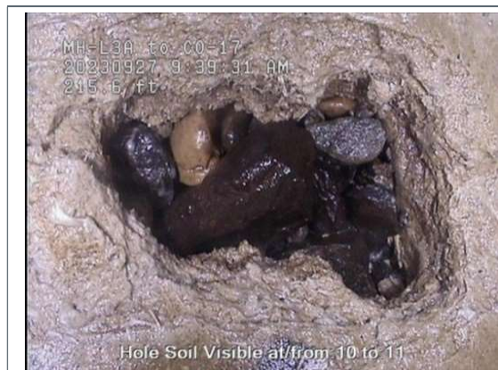
Photo 3. Hole/Broken with Voids Visible
